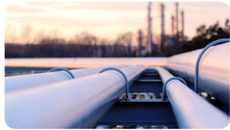
Gas transportation pipeline
