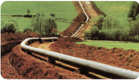
Cross country pipeline
